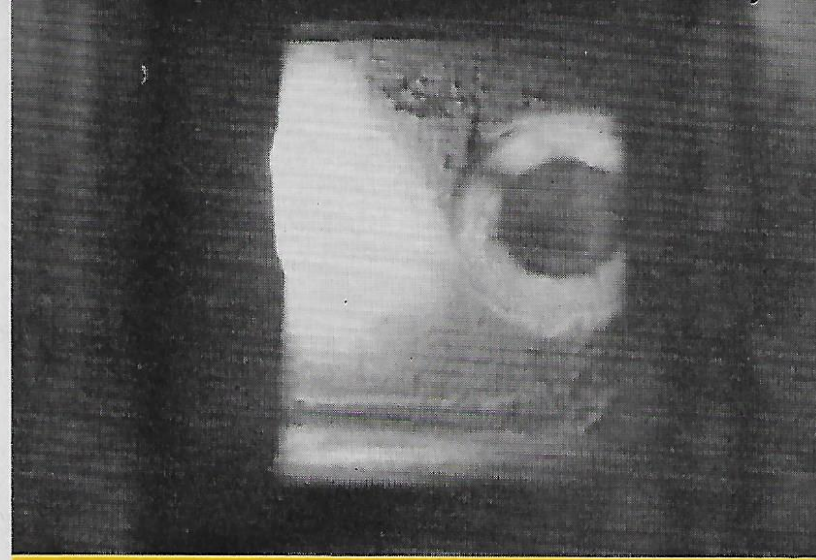
One of several visible evidences of the refinery on stream again is had by glancing into this cracking-heater fire box of Unit 33.
